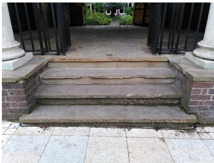
From St John's Square to the Priory Gallery there are four ascending steps. There are no handrails.
